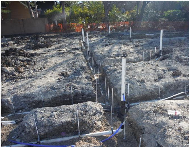
Rough Plumbing with hanging pipe brackets and threaded rod to penetrate the slab
