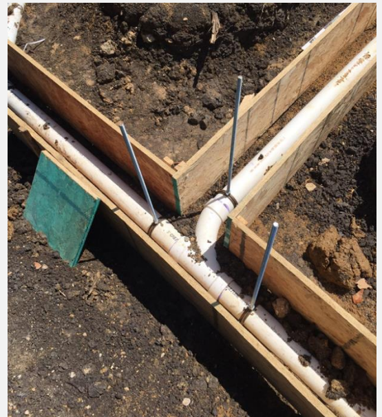
Rough Plumbing with hanging pipe brackets / threaded rod. The void is formed with plywood forms.
