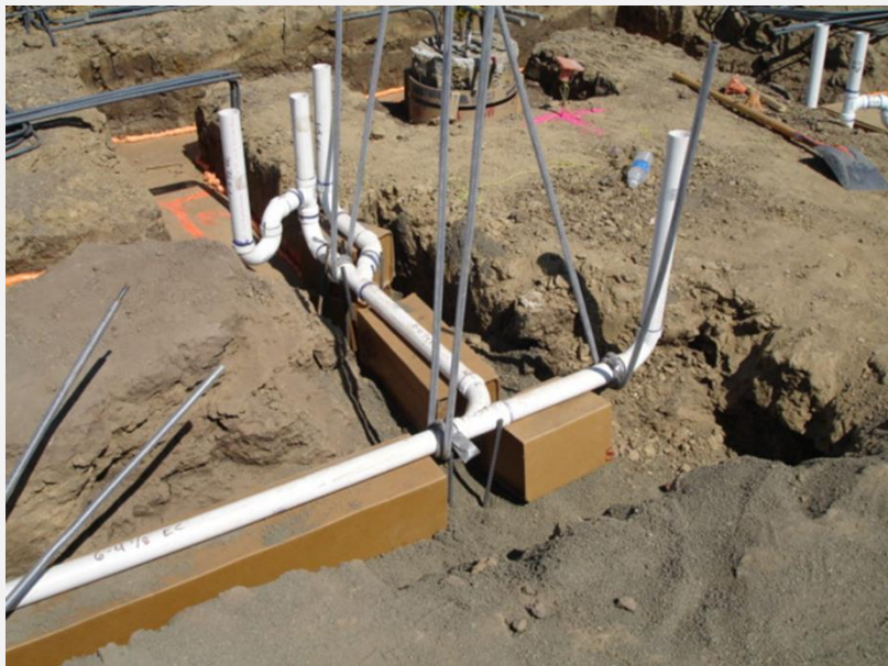
Rough Plumbing placed entirely on top of void boxes and suspended plumbing conduit stakes
