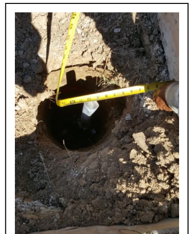
The Helical Pier is measured to assure it is center and cut to the proper height
