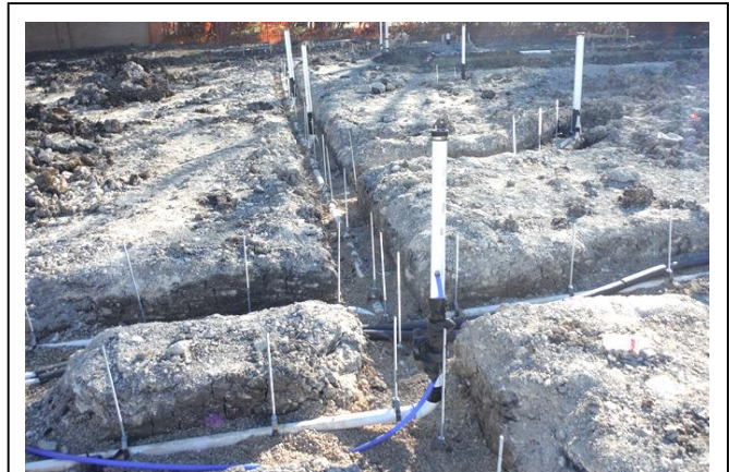
Suspended Plumbing with Threaded Rod
