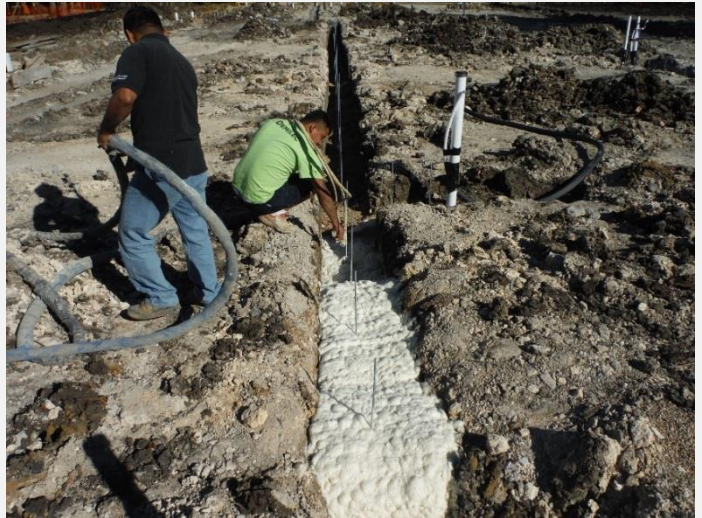
Void between top of plumbing and bottom slab filled with lightweight foam to enable easy lifting of plumbing with slab lift
