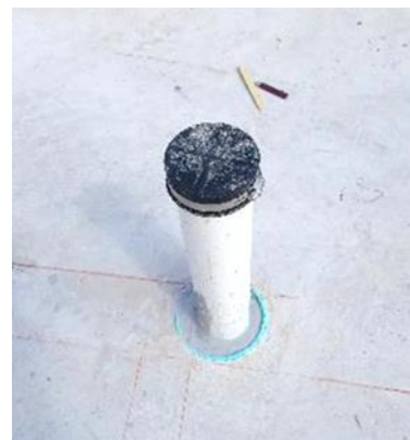
Stack Grouted Flush with Slab
