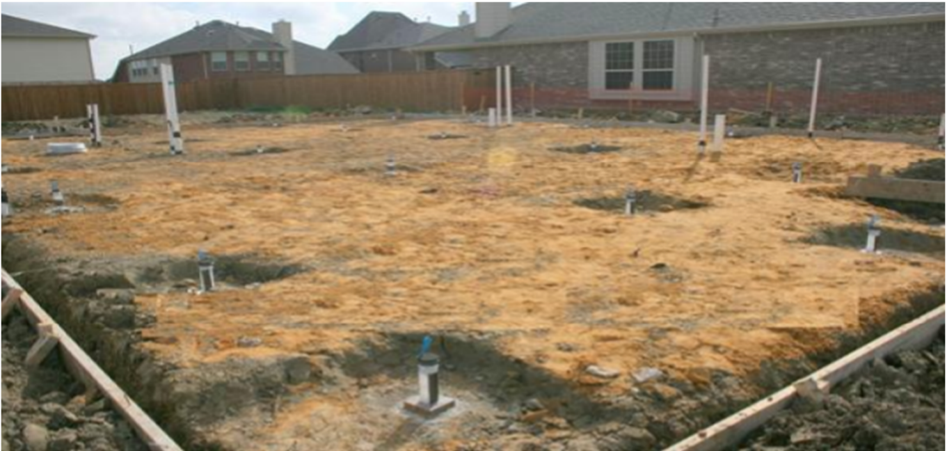
Piers, Mechanisms, Capitals, Perimeter Beams, Pad prepared – ready for installation of reinforcement
