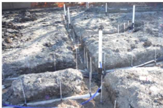
Suspended Plumbing with Threaded Rod
