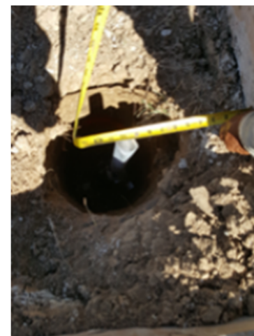
The helical pier is measured to assure it is center and cut to the proper height
