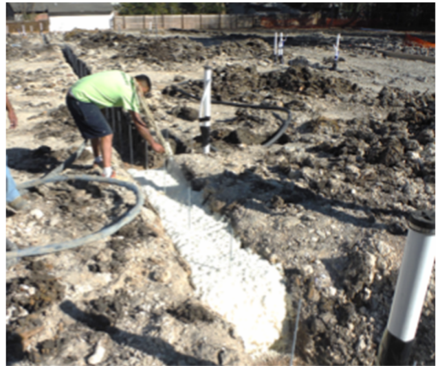
Suspended Plumbing with light-weight material covering plumbing prior to the slab pour and slab lift
