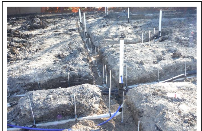
Suspended Plumbing with Threaded Rod
