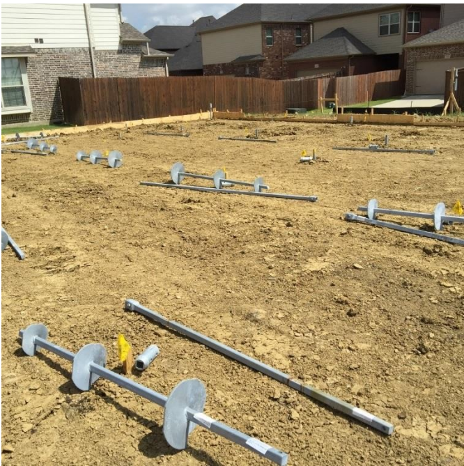
Triple-Helix Helical Piers are laid out on the job site in preparation for installation.
