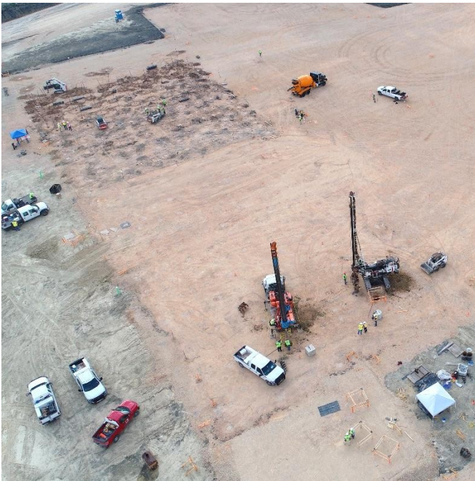
Helical Piers installed together with heavy concrete piers used to carry the structural load while Helical Piers carry the slab load.
